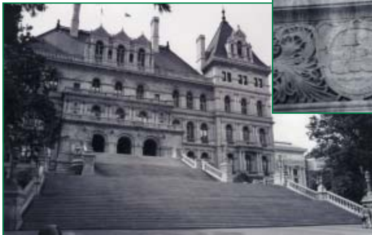
Acid precipitation has taken its toll on New York's finest buildings and monuments. Here, the limestone facade of the NYS Capitol's north side is literally melting away. This shield, and the Port of Albany scene it once depicted, are barely distinguishable, less than a century after the building's construction. A multi-million-dollar rehabilitation project continues on the capitol's exterior. Photos by Gary Randorf.
