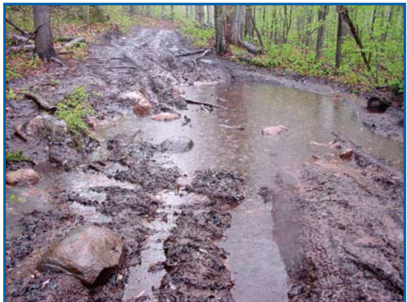
All-terrain vehicle riders have torn up this section of trail in the Aldrich Pond Wild Forest. ATVs are not allowed on Forest Preserve foot trails, but operators often ignore signs and physical barriers erected to keep them out. They cause erosion, wildlife habitat damage, air pollution and water pollution throughout the Adirondack Park.
