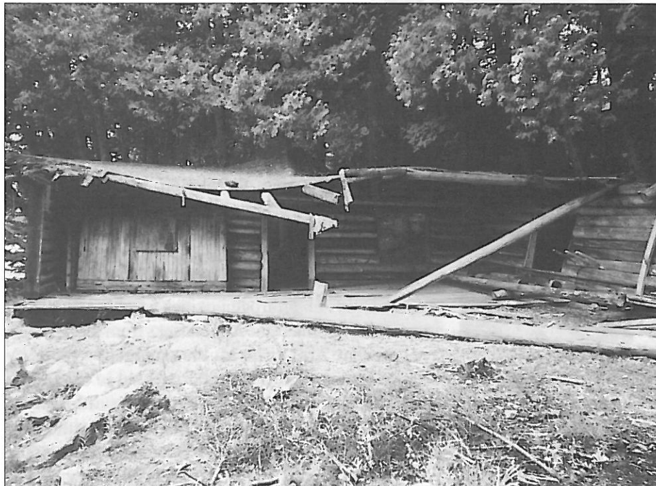
This ramshackle skeleton is all that remains of the boat house at Camp Santanoni. While reconstruction of fallen buildings is not allowed on the Forest Preserve, DEC plans to rebuild and re-use it, claiming that the project is merely "maintenance." Photo by Gary Randorf.
