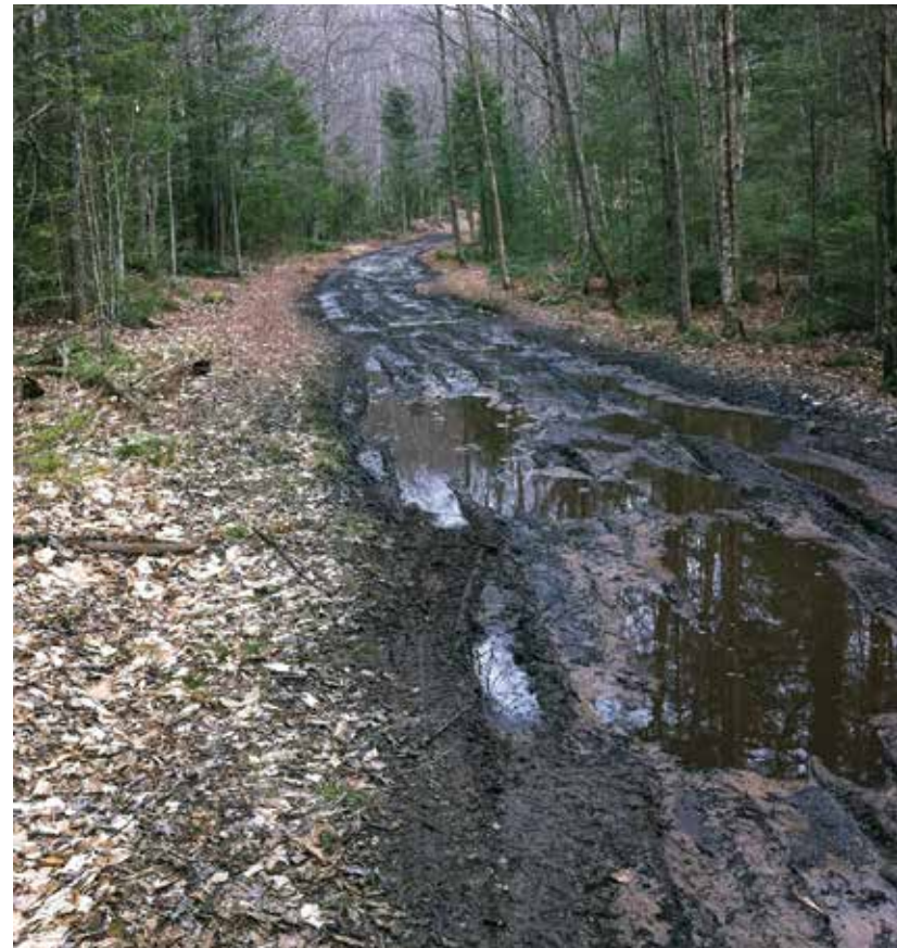
Trail damage in the Independence River Wild Forest
